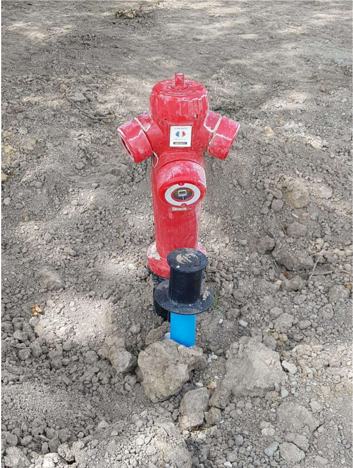
Poteau incendie privé - MENUT ST CYR-EN-VAL
